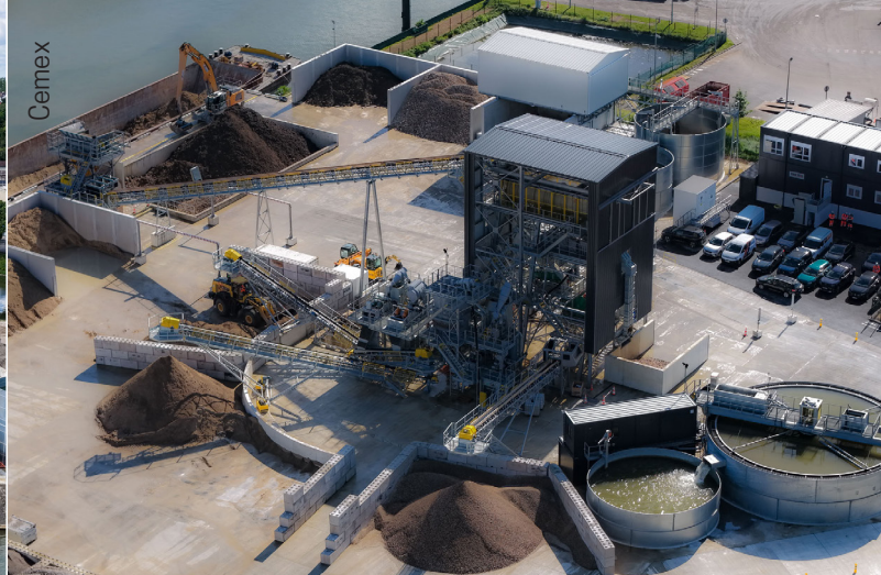
Installation de criblage
